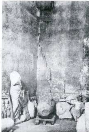
Fig. [56]: The pattern of wall cracks in one of the internal walls.
