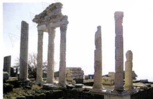
Fig. [43]: A contre-jumière photograph showing clearly the state of displaced drums of the columns on the Acropolis of Pergamon with their edges missing.
