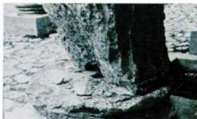
Fig. [11]: Characteristic damage to columns of the Temple of Zeus at Aizani caused the deliberate hewing off of its bottom drum for the lead of its dowel.
