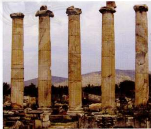
Fig. [14]: A column (No. 2) of the peristasis of the temple of Aphrodite at Aphrodisias, showing incipient failure of one of its drums.
