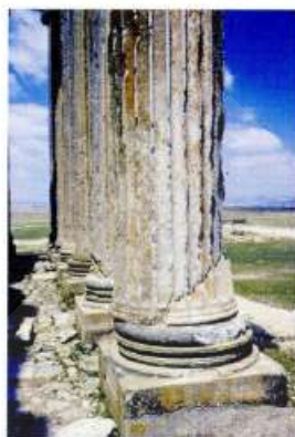
Fig. [9]: Concrete repair corner pillows of bottom drums of the temple of Zeus at Aizani detached from their columns due to their rocking caused by the earthquake of 1970.
