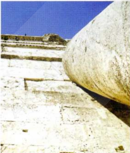
Fig. [21] The column of the south peristyle of the Temple of Bacchus leaning against the cella wall of the temple, which was damaged in arresting its fall.
