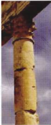
Fig. [13]: Typical damage of drums of the Colonnade near the northern baths in Apamea.
