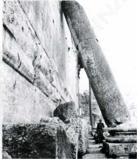
Fig. [20] Column of the south peristyle of the Temple of Bacchus in Baalbek thrown onto the cella wall of the Temple by the earthquake of 25 November 1759.
