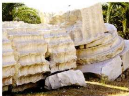
Fig. [40]: Corner failure of the bottom drum of the column; the missing piece lies on the ground.
