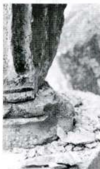
Fig. [10]: Typical corner fracture of the lower part of bottom drums of columns of the Temple of Zeus at Aizani due to rocking caused by the earthquake of 1970.
