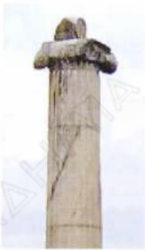
Fig. [3]: Diagonal cracks of drums.
